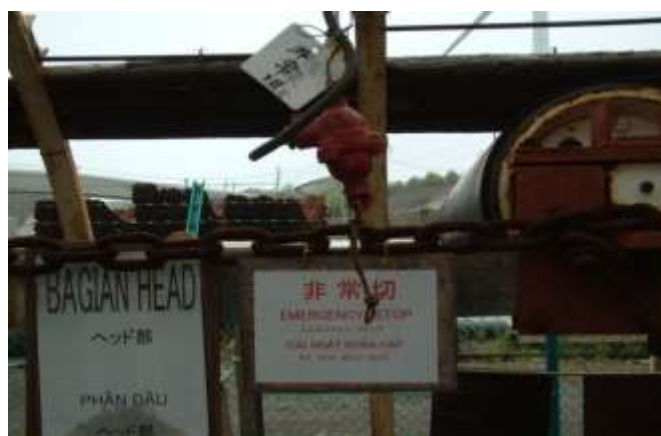
Gambar 15 Tali Emergency Switch
